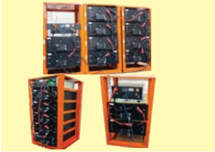
Energy Storage System (ESS)
